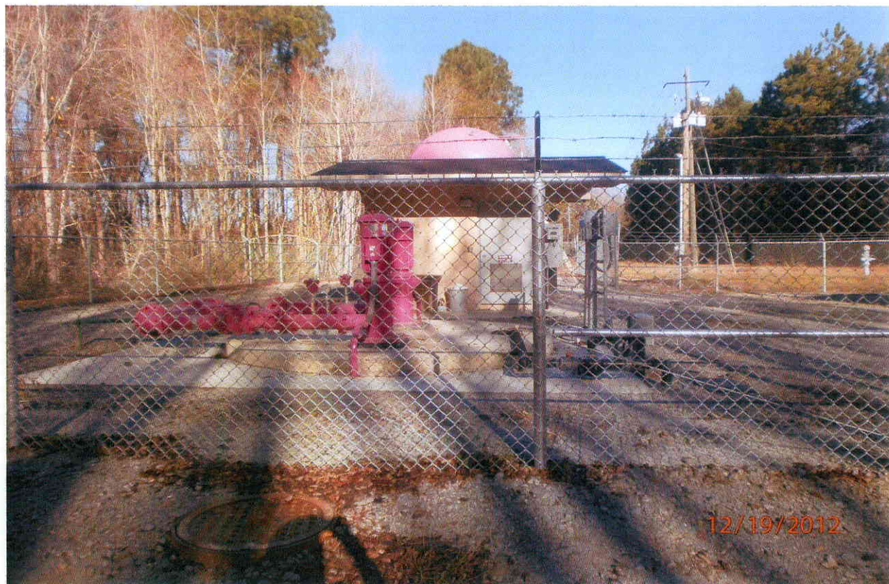
Figure 3: City of Statesboro Lift Station with Purple Pipes.
