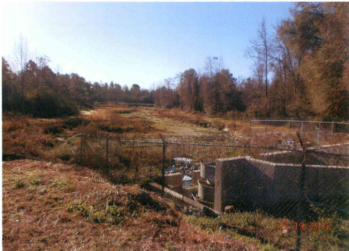
Figure 5: Waste Water Aerator.
