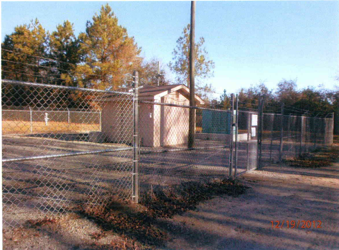
Figure 4: City of Statesboro Lift Station.
