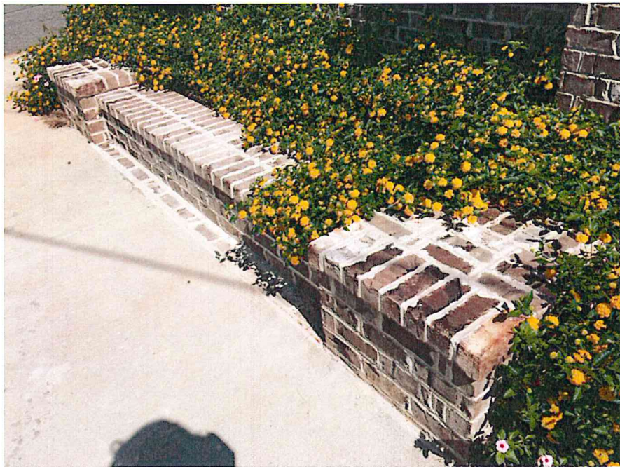
Picture 4 Installation 8" up to Property Line on Left Side of Sign (Upper Corner of Picture)
