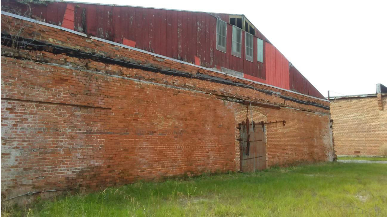
Picture 5 Exterior Entrance Depicting Adjacent Warehouse at 20 East Vine Street in far Right Corner
