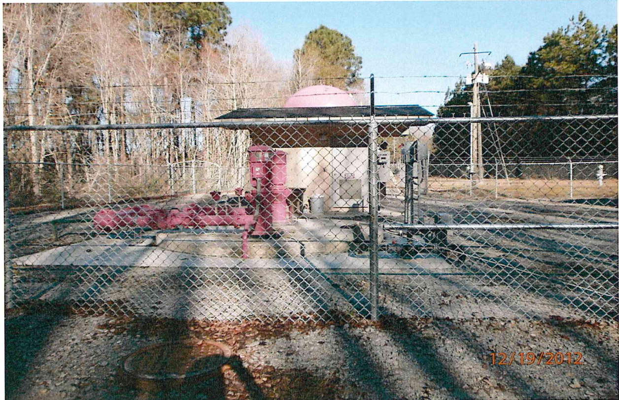
Figure 3: City of Statesboro Lift Station to the south abutting the Subject Property.
