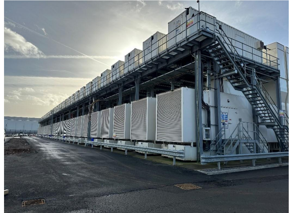
Photo Credit: WB Power Solutions
