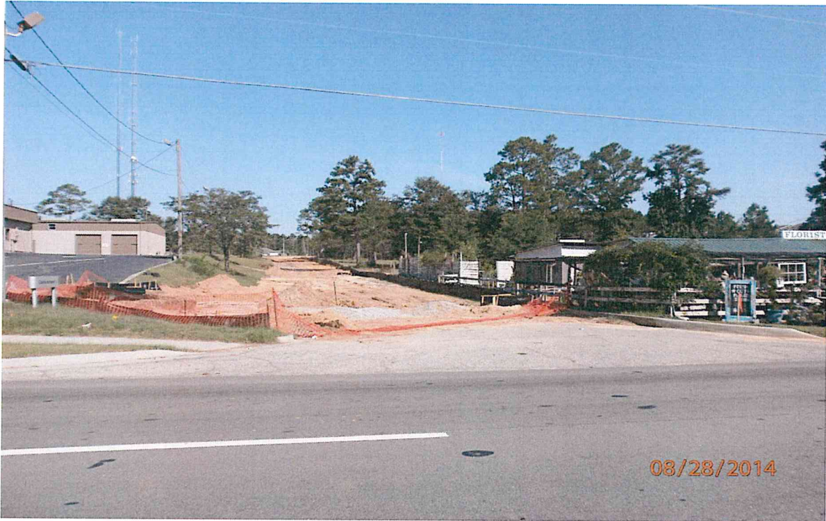
Figure 5: Access road being built connecting Highway 301 with the subject property to be deeded to the City of Statesboro as public right of way.
